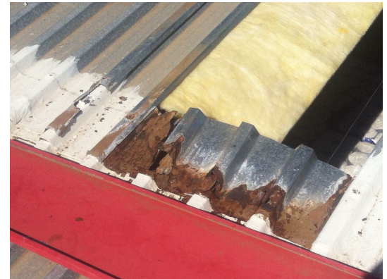
Failing end lap detail that had no sealant tape
