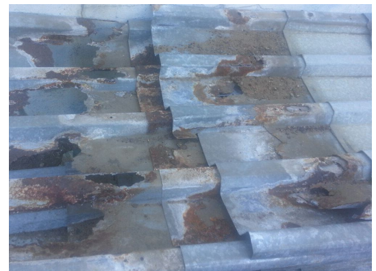
Corroded end laps on IBR roof sheeting
