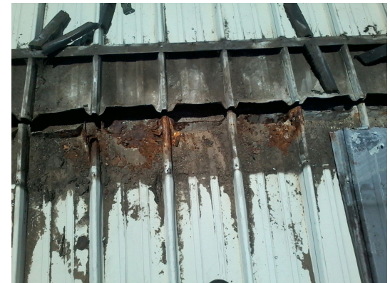
Corrosion of roof sheet as a result of moist debris build-up
