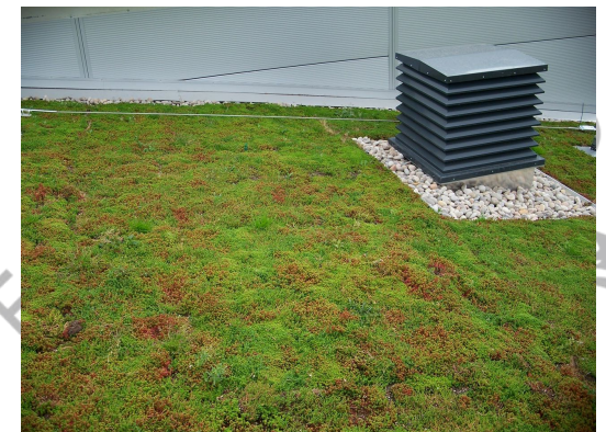
Penetration and drains protected by retention rails
