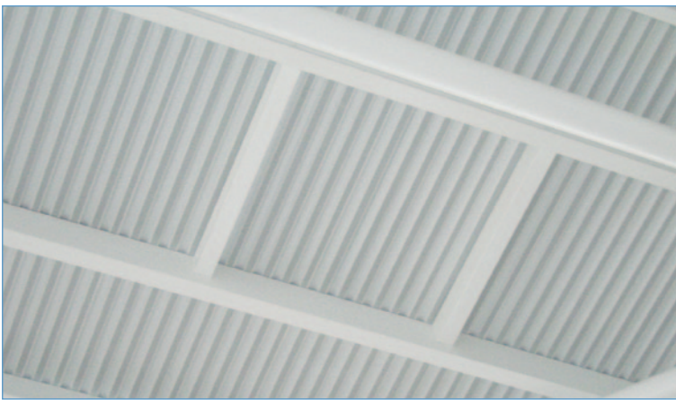
Internal view of the sealed white Walkable Liner Sheet.
