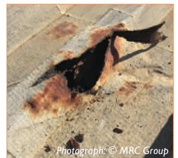
Water vapour sealed within the end lap by the waterproofing has accelerated the corrosion process.
