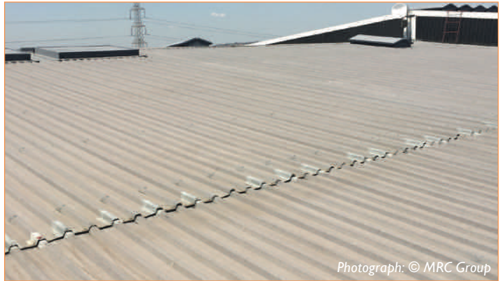
Failed open end lap, allowing the ingress of wind-driven rain.
