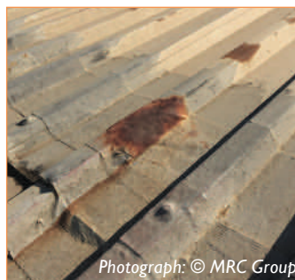
Breakdown of the end lap from rust under the waterproofing.
