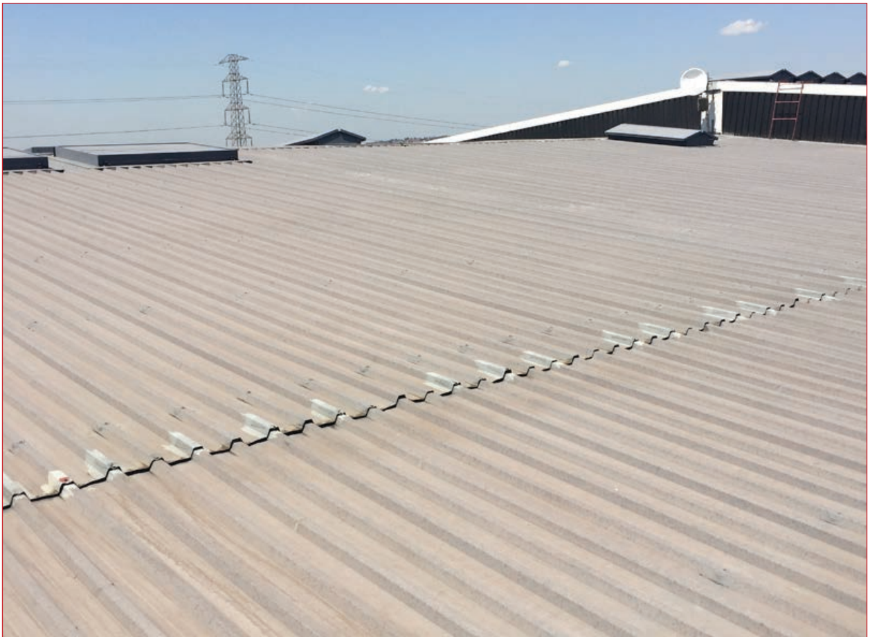
A failed end lap.
