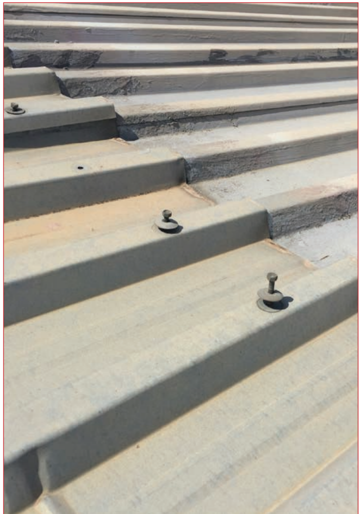
Loose screws, due to thermal expansion.
