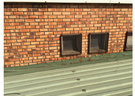
Failed metal flashing with waterproofing
