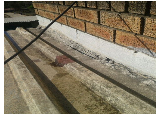
Failed waterproofing membrane and no metal flashings
